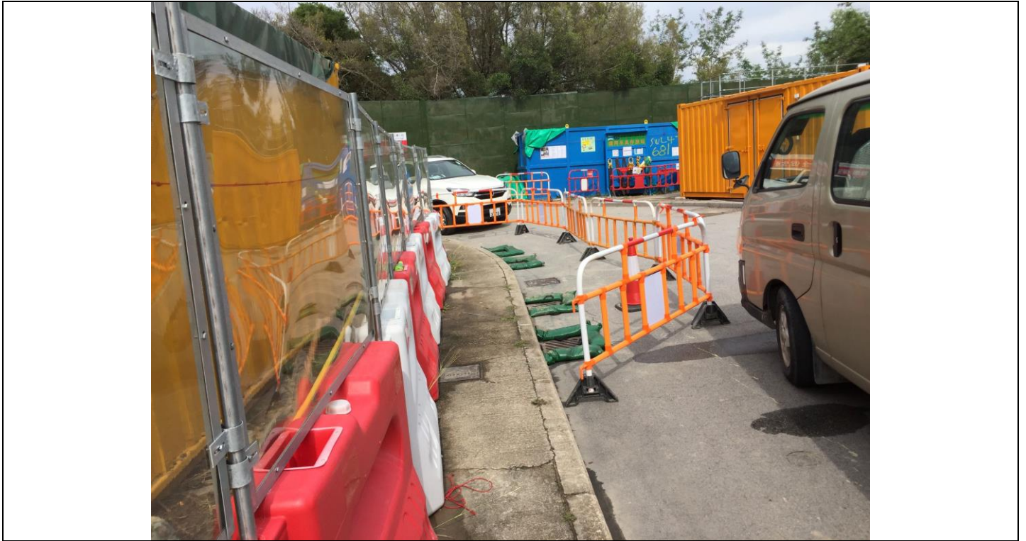
Date of site inspection: 25 May 2021 Gullies were banded by sand bags to prevent surface runoff.
