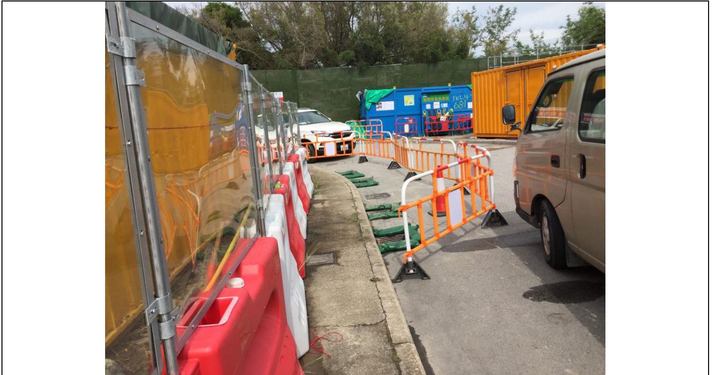
Date of site inspection: 25 May 2021 Gullies were bunded by sand bags to prevent surface runoff.
