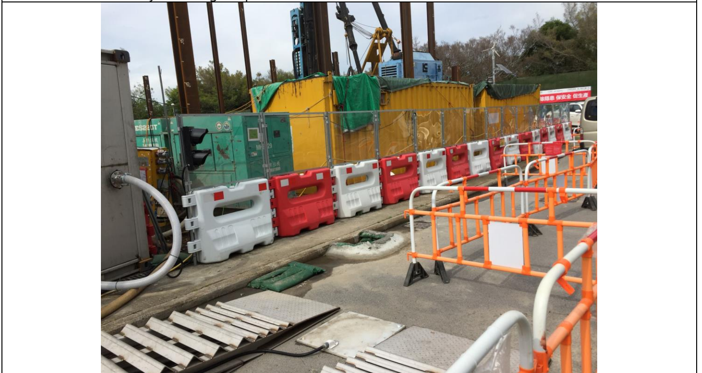
Date of site inspection: 25 May 2021 The surrounding of gullies near the construction site areas were temporarily sealed.
