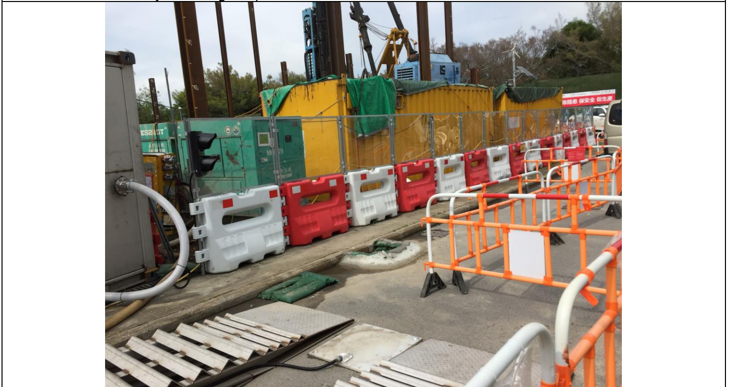
Date of site inspection: 25 May 2021 The surrounding of gullies near the construction site areas were temporarily sealed.
