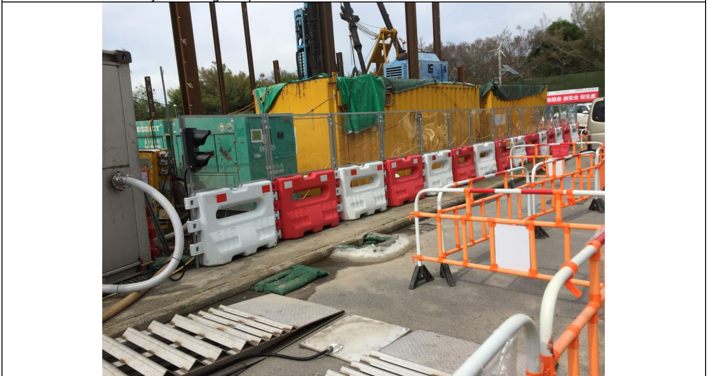
Date of site inspection: 25 May 2021 The surrounding of gullies near the construction site areas were temporarily sealed.
