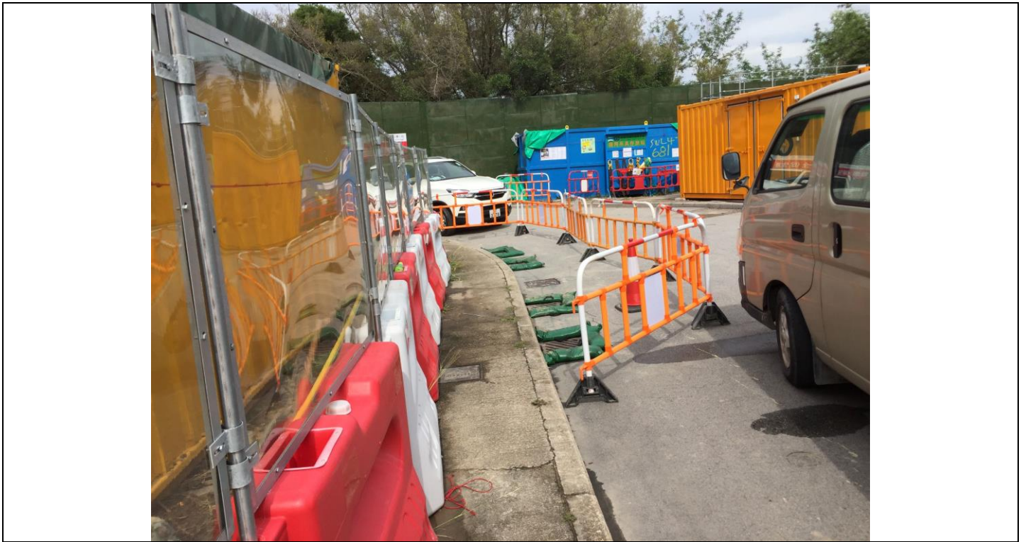
Date of site inspection: 25 May 2021 Gullies were banded by sand bags to prevent surface runoff.
