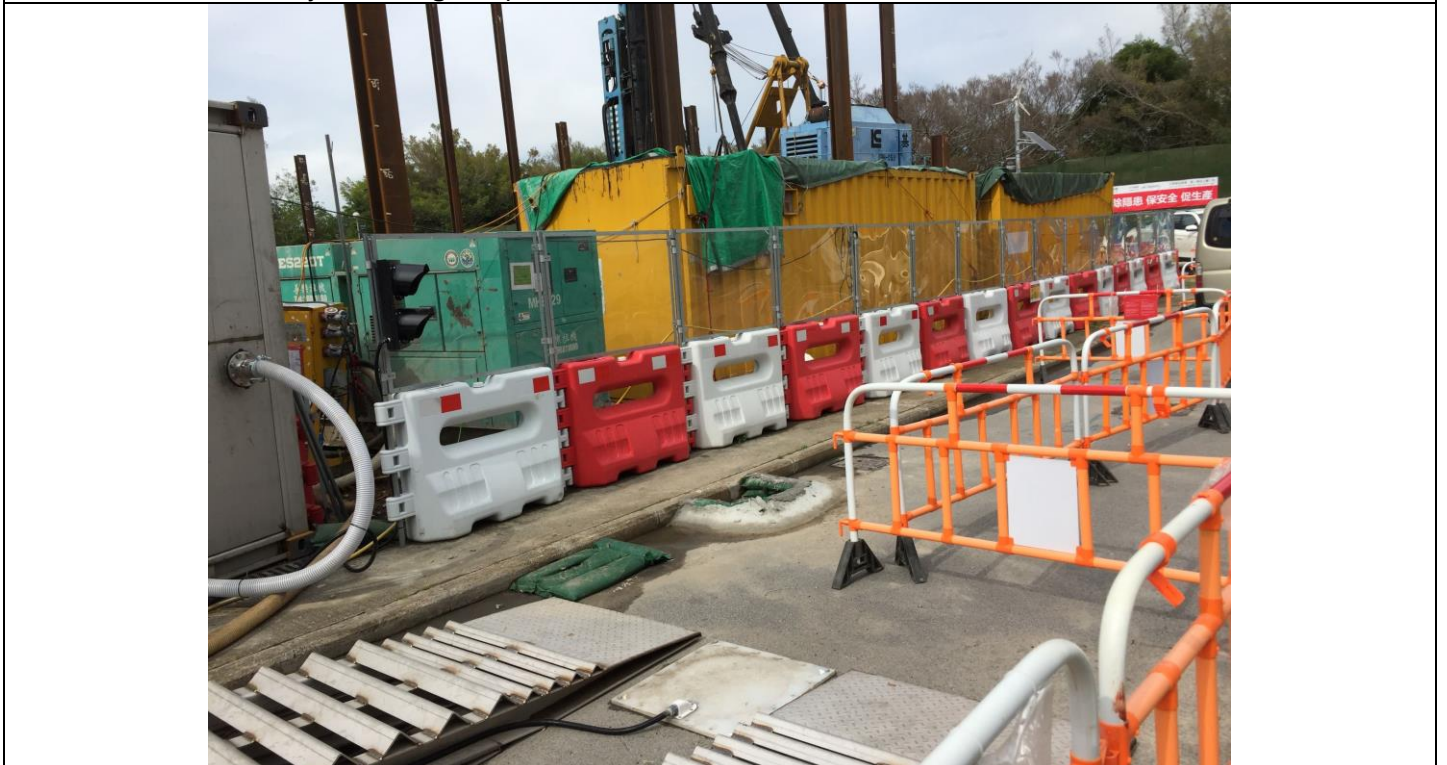
Date of site inspection: 25 May 2021 The surrounding of gullies near the construction site areas were temporarily sealed.
