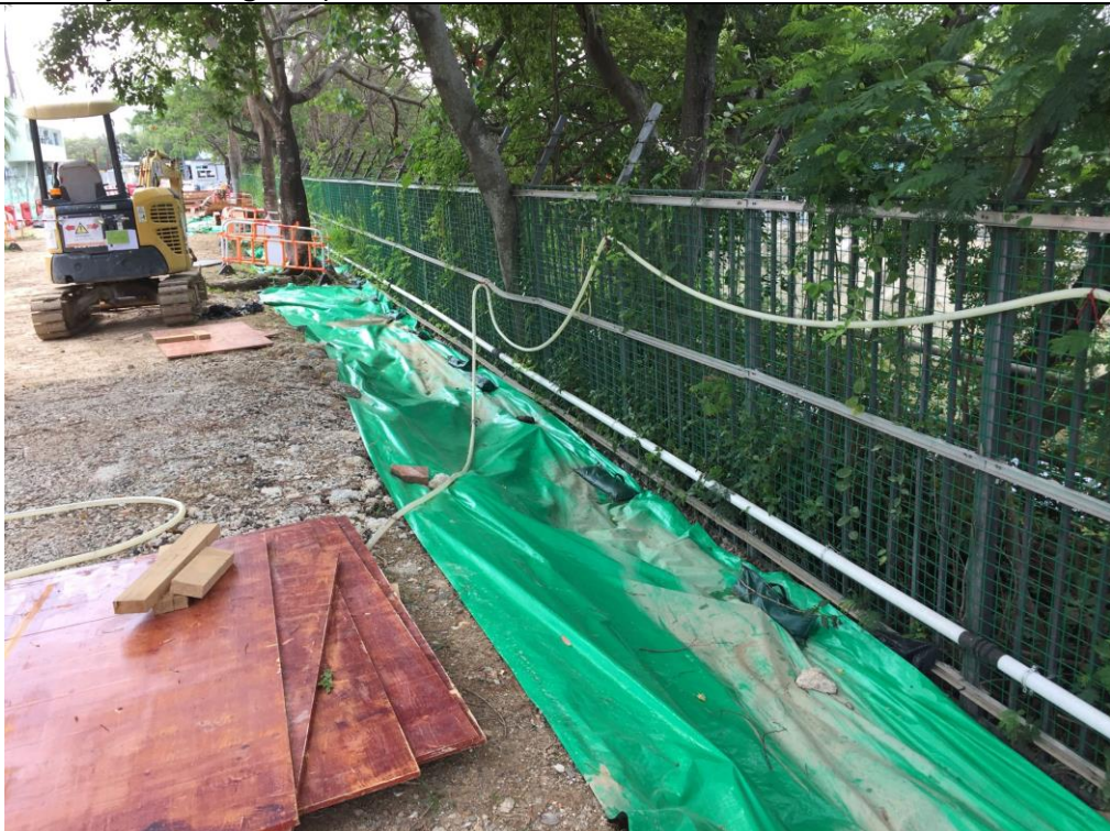
Date of site inspection: 8 June 2021 The surrounding of the construction site areas were covered by impermeable sheeting to prevent surface runoff.
