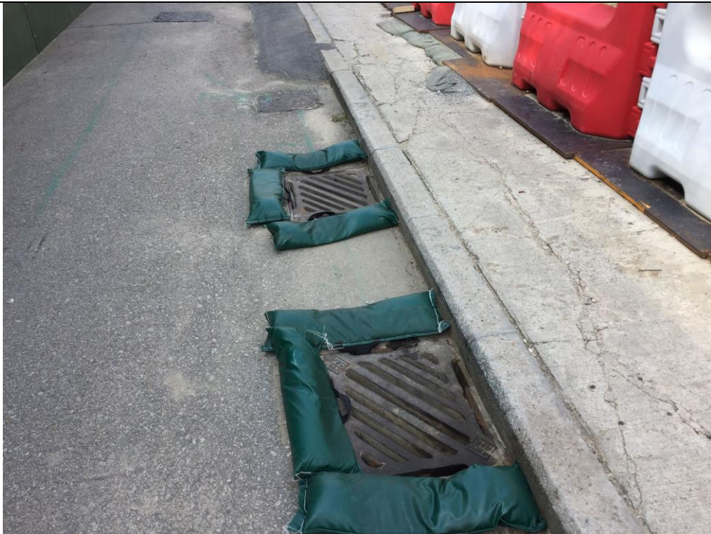
Date of site inspection: 8 June 2021 Gullies were banded by sand bags to prevent surface runoff.
